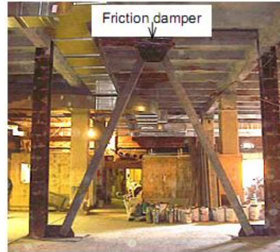
Figure 5. Friction damper at top of chevron brace.
